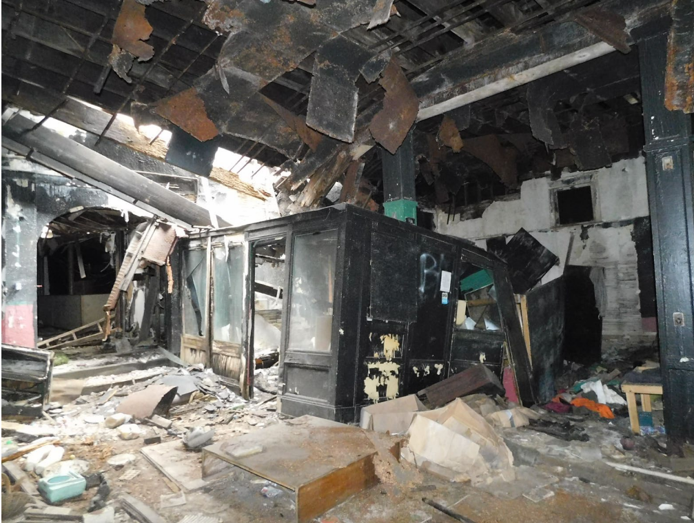
1st floor deck caving into basement
