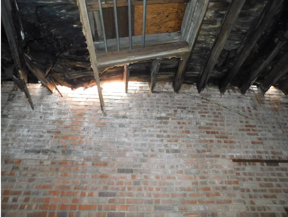
Joints not connected to bearing wall
