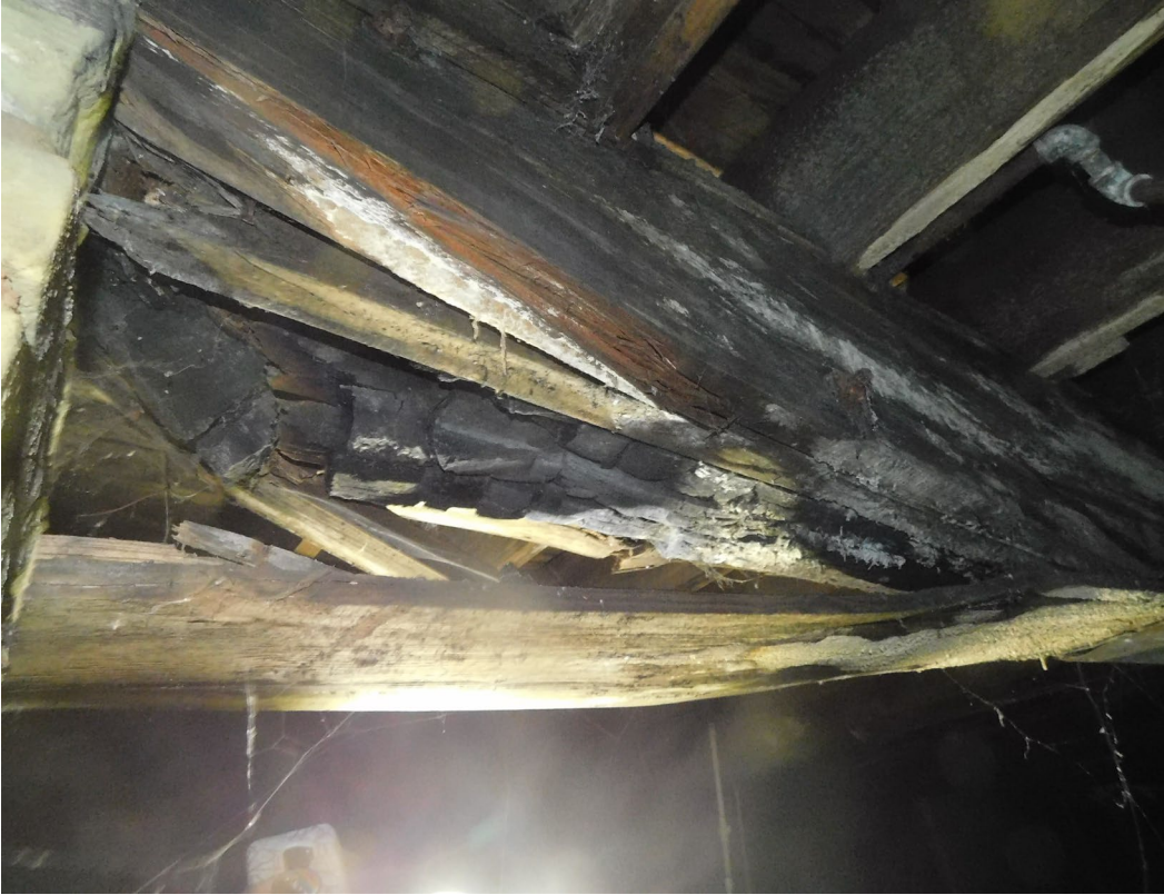
Basement beam burnt
