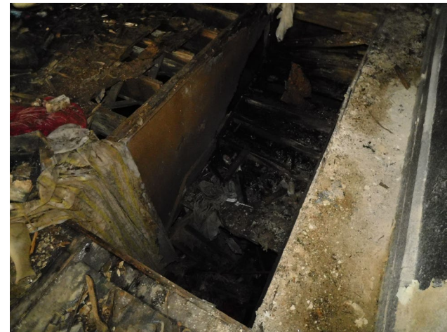
Basement staircase gone
